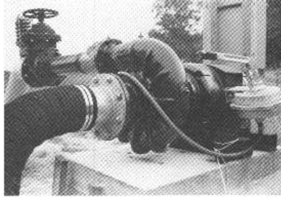
Figure 1. Electric-motor-driven centrifugal pump drawing water from a surface water supply.
