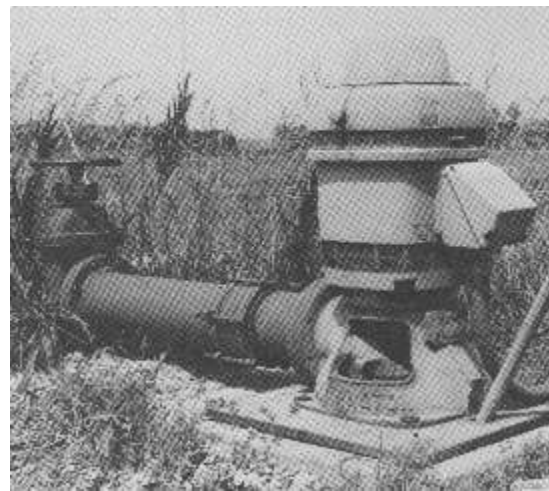
Figure 2. Electric-motor-driven turbine pump drawing water from a deep well.
